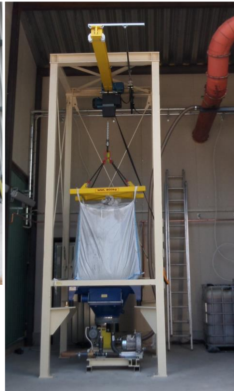
Metering and dosing system
