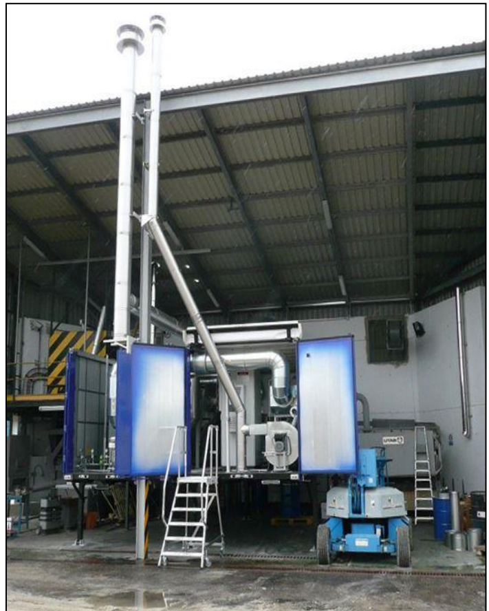
Mobile Ammunition disposal plant: Amunmobil
