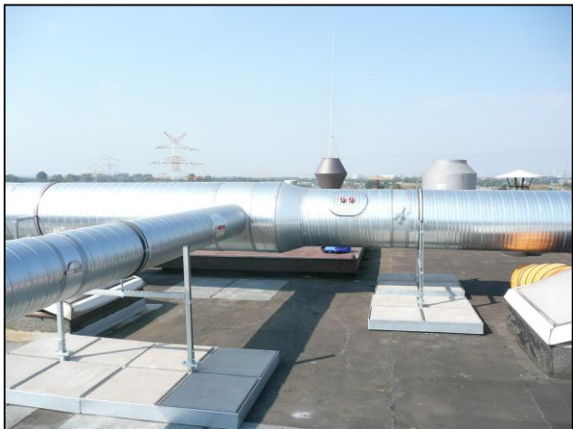
Junction of various exhaust air ducts
