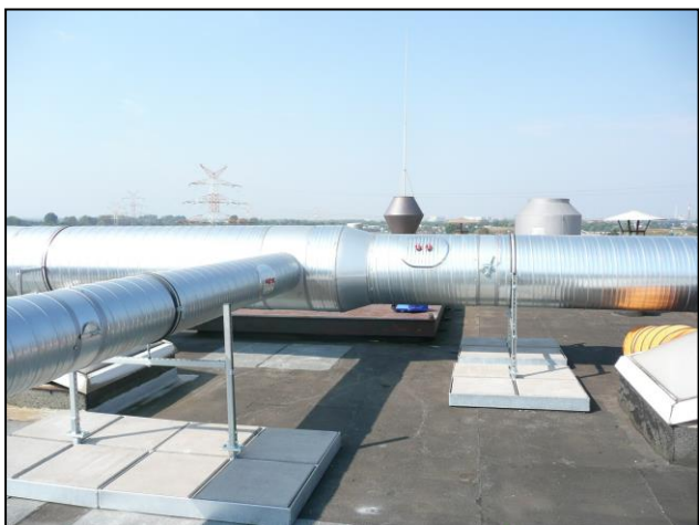
Junction of various exhaust air ducts
