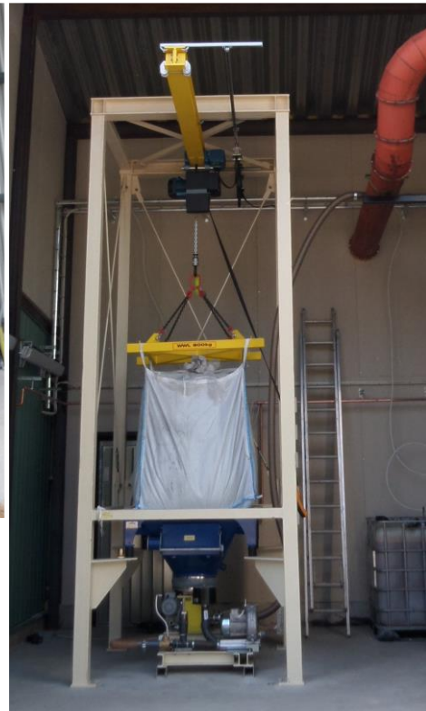
Metering and dosing system
